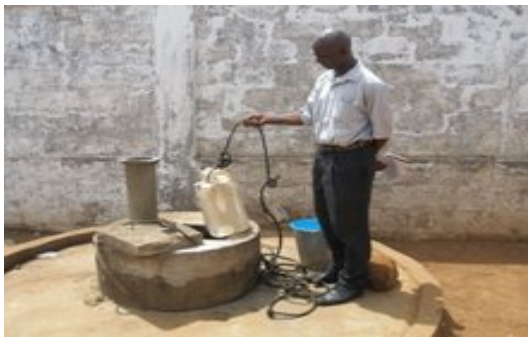
A teacher at King Elementary School uses a worn plastic bucket to haul drinking water from a broken well—the only source of drinking water for students.
